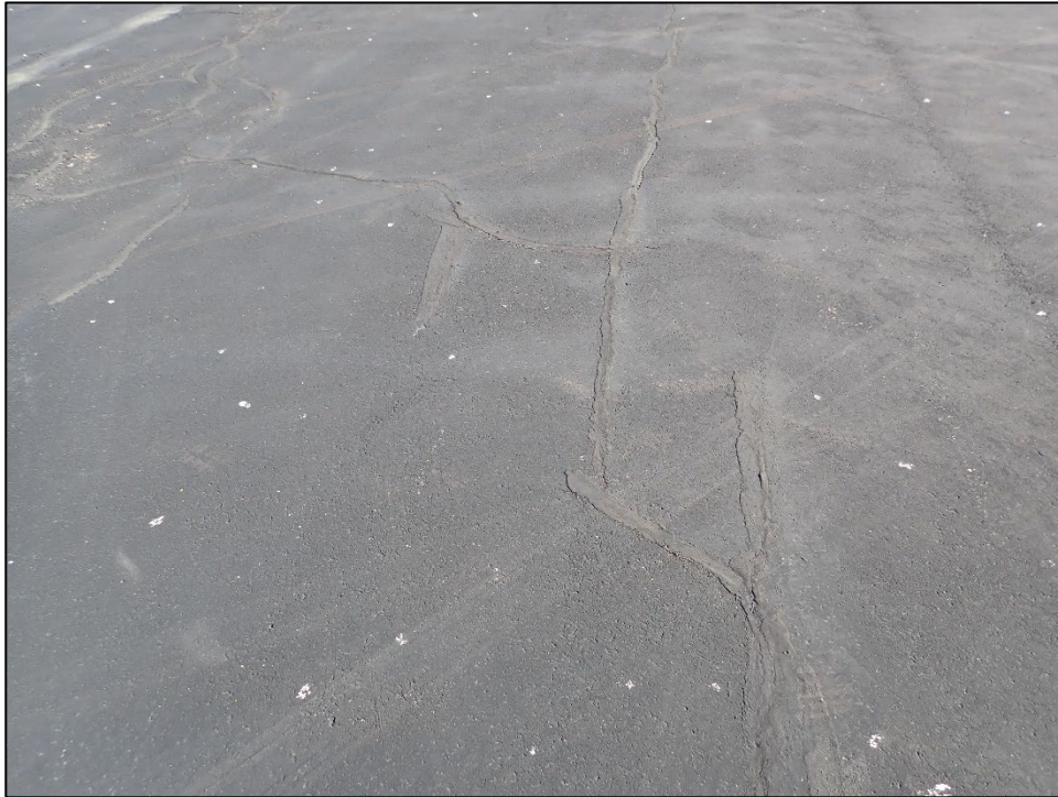
AP-11-01: L&T Cracking
