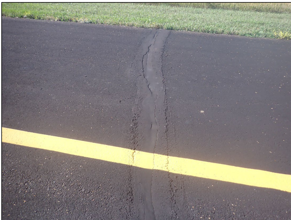
TW-13-02: L&T Cracking
