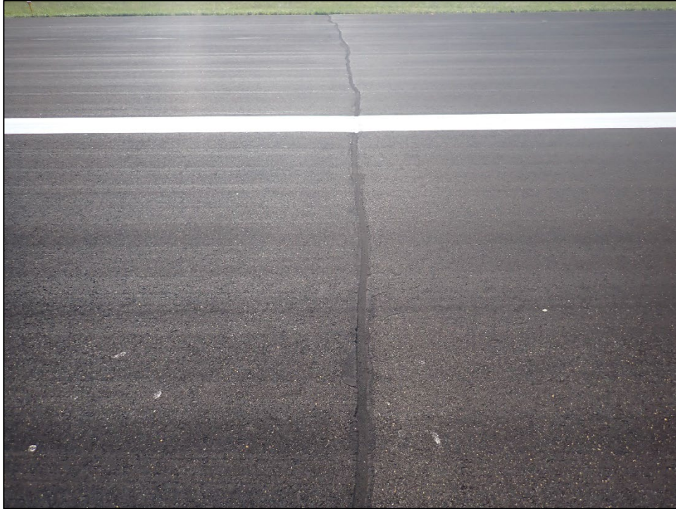
RW12-11-31: L&T Cracking
