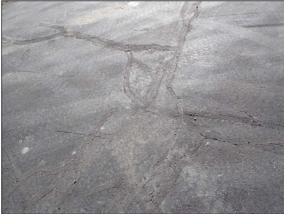
TW-11-06: L&T Cracking
